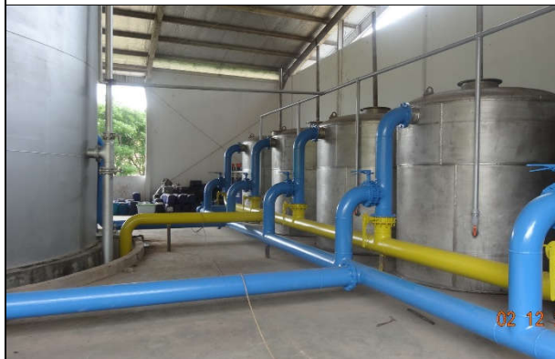
Water Treatment Purifier
