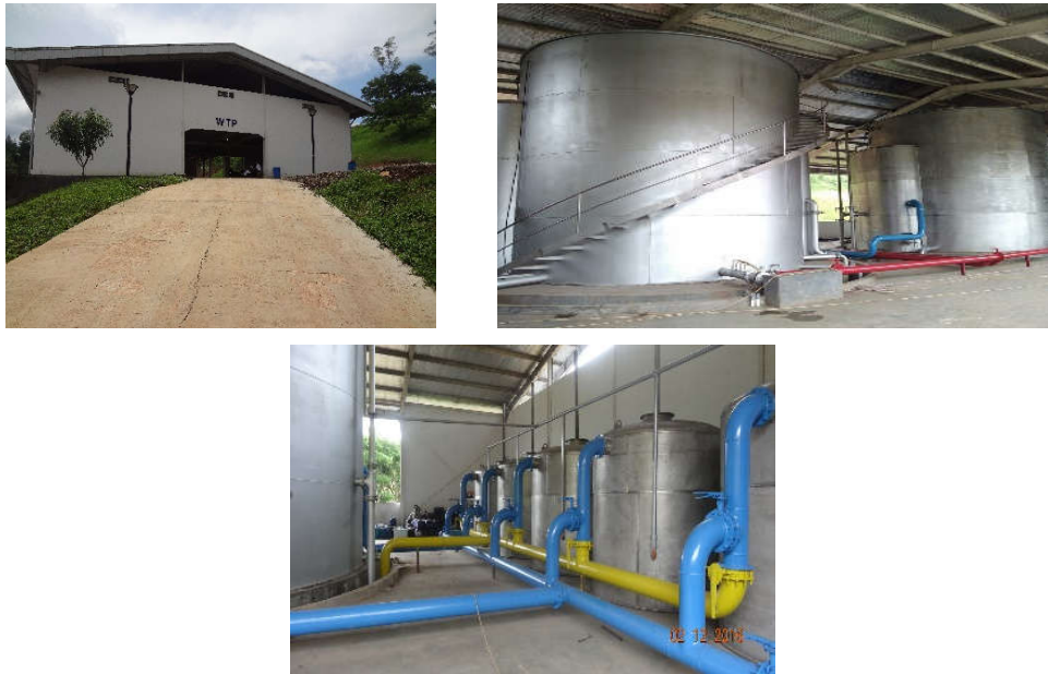
Gambar 3.23 Water Treatment Plant (WTP)
